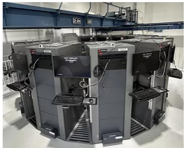
Figure 2: Keysight's 1000-Qubit Quantum Control System solution installed at the National Institute of Advanced Industrial Science and Technology (AIST) in Tsukuba, Japan [3].
